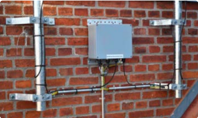
REdY Concentrator 1M mounted on rooftop gable with double antenna
