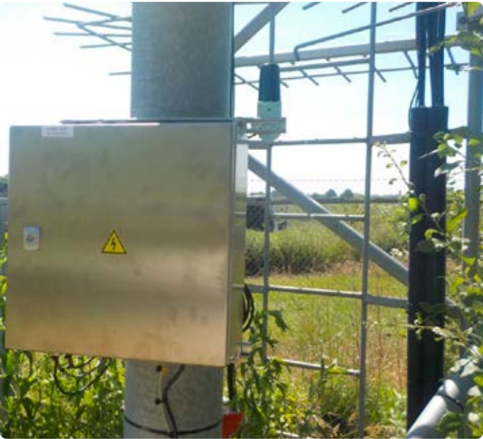
REdY PSU-4 mounted at street level
